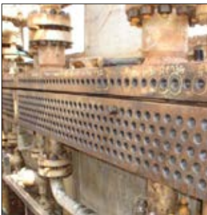
FinFan cooler before a maintenance
